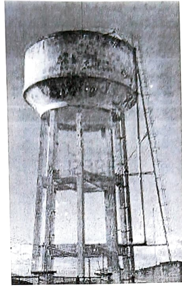
Fig. 1.4(B) Intake water Tank
